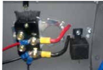
UNCOVERED-Location of relay
