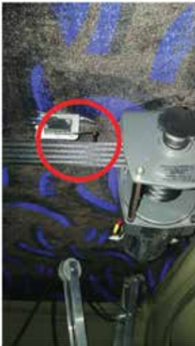
Location of Limit Switch near the winch motor
